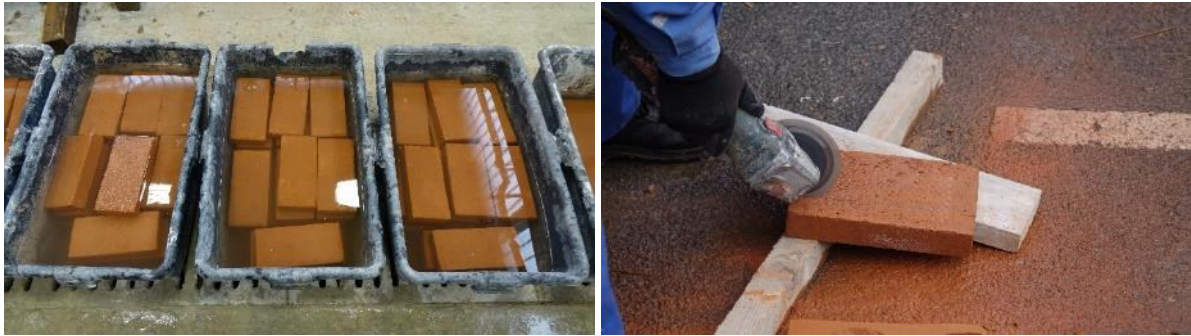
Fig. 14: Soaking the bricks before laying (left) and cutting by a circular saw (right).
