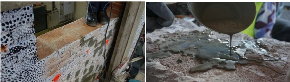
Fig. 20: Drilling the holes for the injection (left) and gravitational injection of the wall (right).
