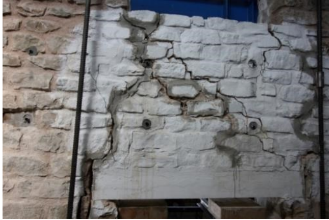
Fig. 107: Damage on the unstrengthened side after the test.
