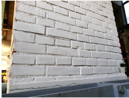
Fig. 87: Cracks on the unstrengthened side at u=-22.0 mm
