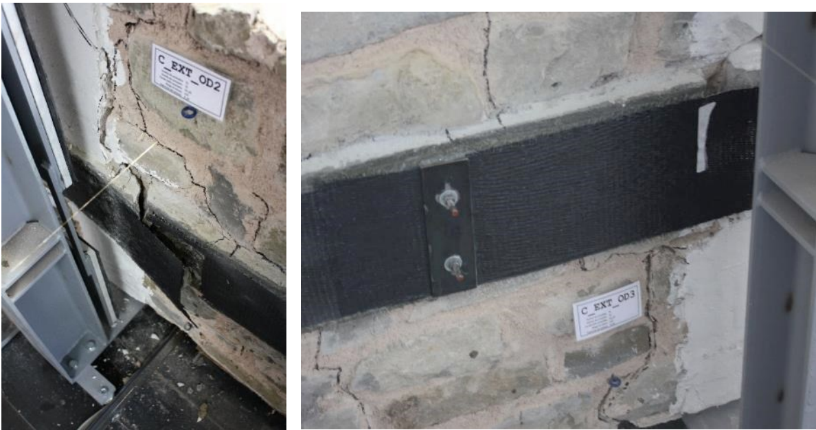
Fig. 170: crack configuration during the test – (a) unreinforced side middle section at step 2 (-0.58 mm); (b) unreinforced side middle section at step 7; (c) reinforced side middle section at step 7
