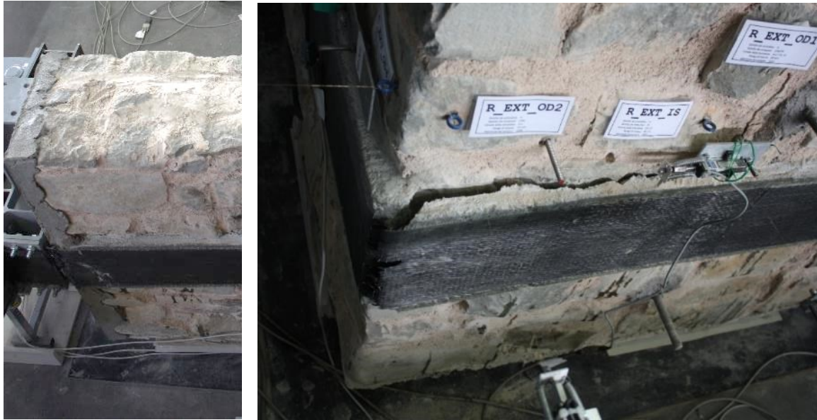
Fig. 172: (a) Detachment and partial breakage of the FRP strip from the masonry at the left support; (b) breakage of the CFRP strip in the right corner at -45.9 mm
