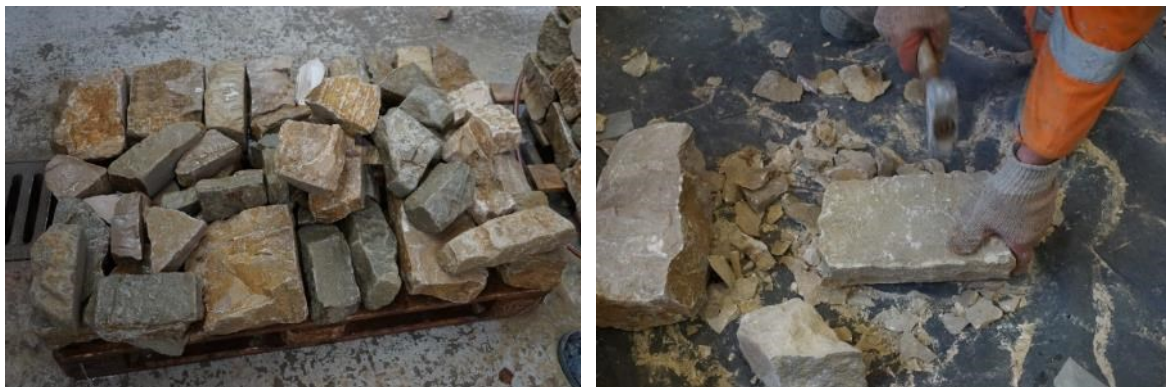
Fig. 1: Sorted stones ready for construction (left) and shaping of stones by hammer (right).
