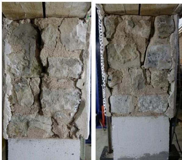
Fig. 116: Separation of wall leaves in piers
