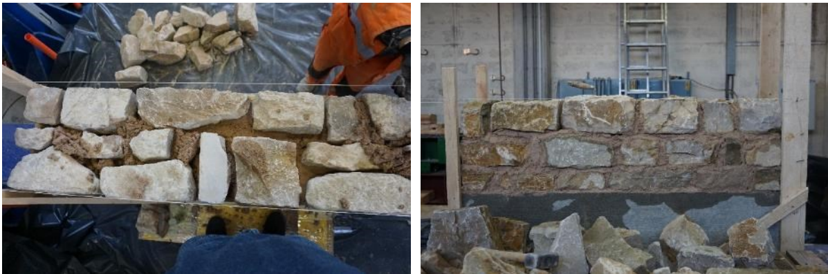
Fig. 9: Stones in two-leaf masonry wall (left). Overlapping of stones between rows (right).
